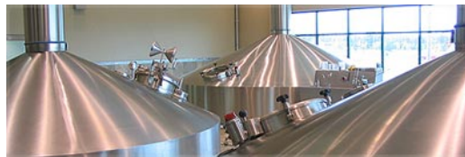
State-of-the-art Huppmann Brew House is energy efficient. With low-NO x burners, the boilers reduce air emissions.
